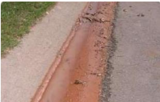
Wastewater residues left in a roadside gutter
