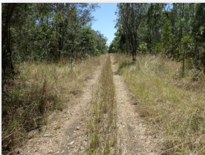
The railway formation through the mining lease is in great condition and is used already by mountain bikers and walkers. Unfortunately, it cannot be used for the trail at this time.
