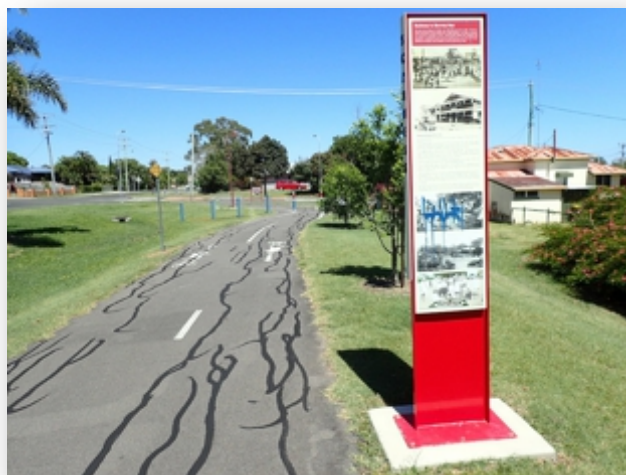
(Above: existing Mobility Corridor) A sealed trail provides access for a greater number of user types (those with road bikes for example) but does present a series of ongoing maintenance tasks especially crack repairs.
