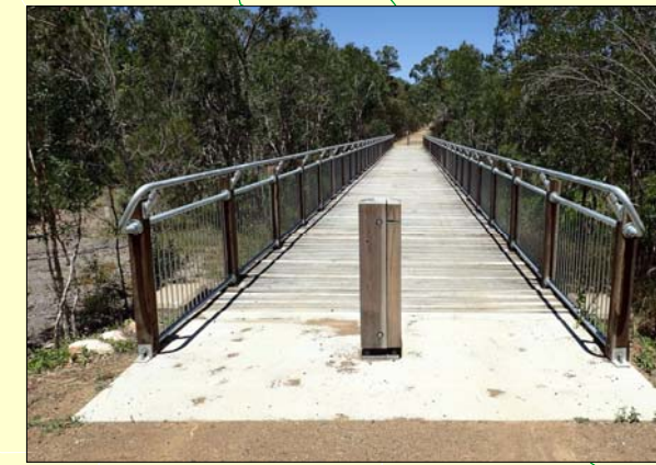
One of the new pedestrian/cyclist bridges constructed on the recently opened section of the rail trail.
