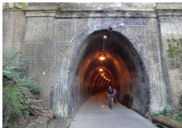
Above: The Fernleigh Track in Newcastle is exceedingly popular with a range of users. One of its key attractions is the Fernleigh Tunnel.
