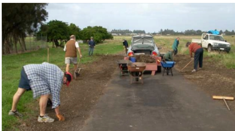
Volunteers organised by the Committee of Management at a busy bee to undertake maintenance work along the rail trail near Port Fairy in western Victoria.
