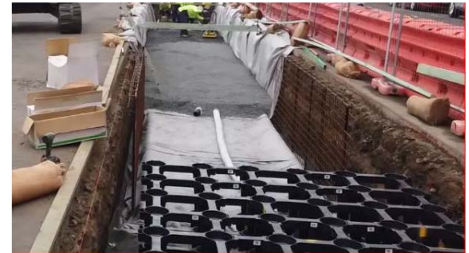
FIGURE 10 : StrataVault system tree trench installed in a roadway, Inverell, NSW 2018. Image courtesy of Citygreen.
