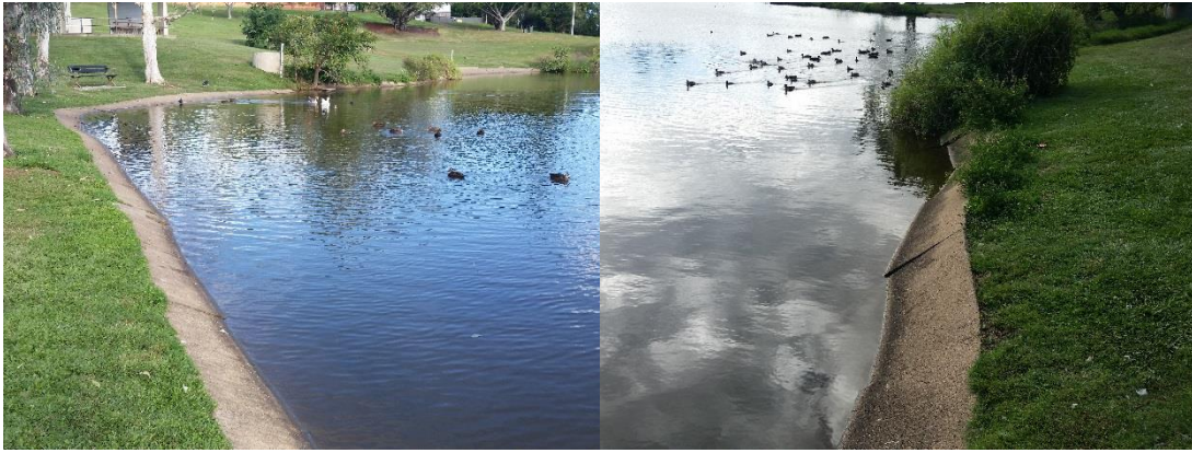
Figure 4-1 Concrete revetment in the SE corner of Ululah Lagoon: a) Main section, and b) Collapsed section towards the northern end.
