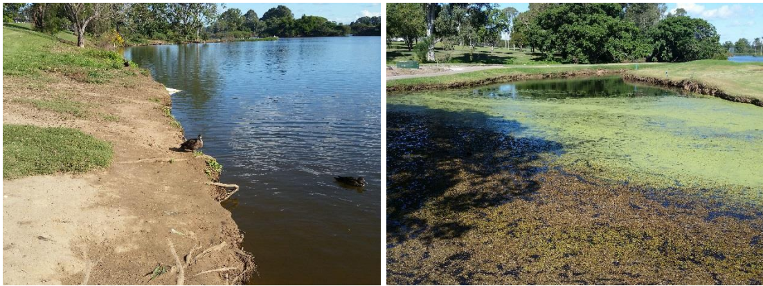
Figure 4-2 Minor scour present below grassed edges creating shallow vertical edge.
