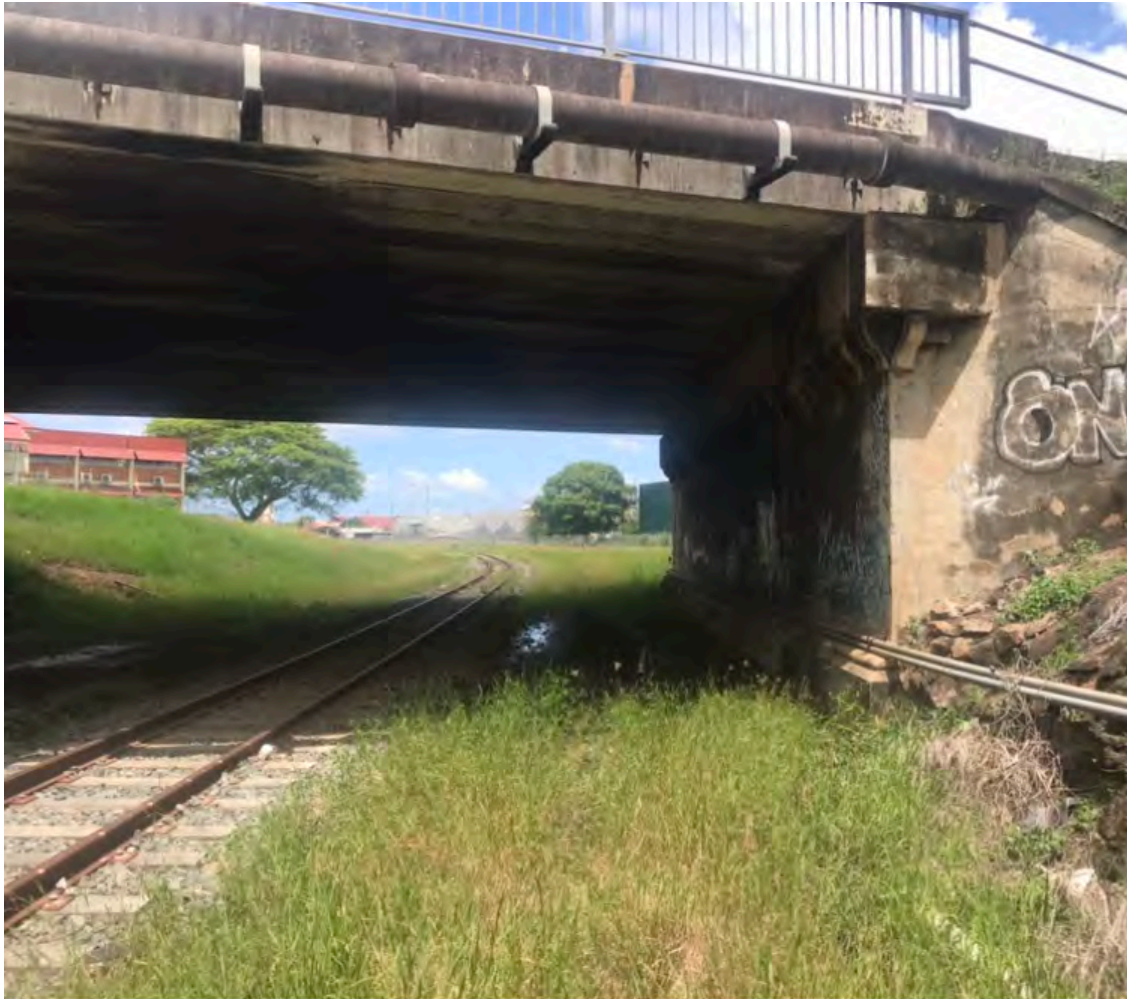
18. Ferry Road underpass - 2m+ gap between bridge support and edge of sleepers.
