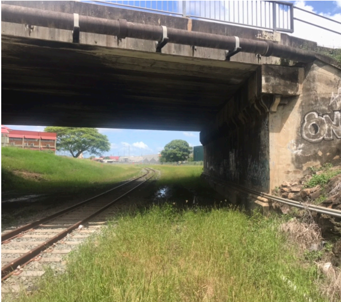
18. Ferry Road underpass - 2m+ gap between bridge support and edge of sleepers.
