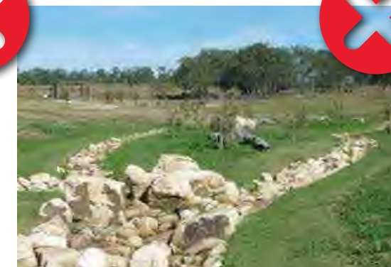
Dumped rock - poor ecological function, prone to weed infestations, difficult to maintain without using herbicides in waterway
