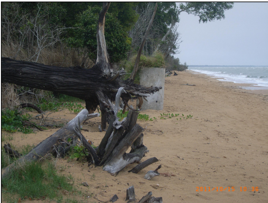
Figure 6.2: Fallen Vegetation and Exposed Drainage Infrastructure
